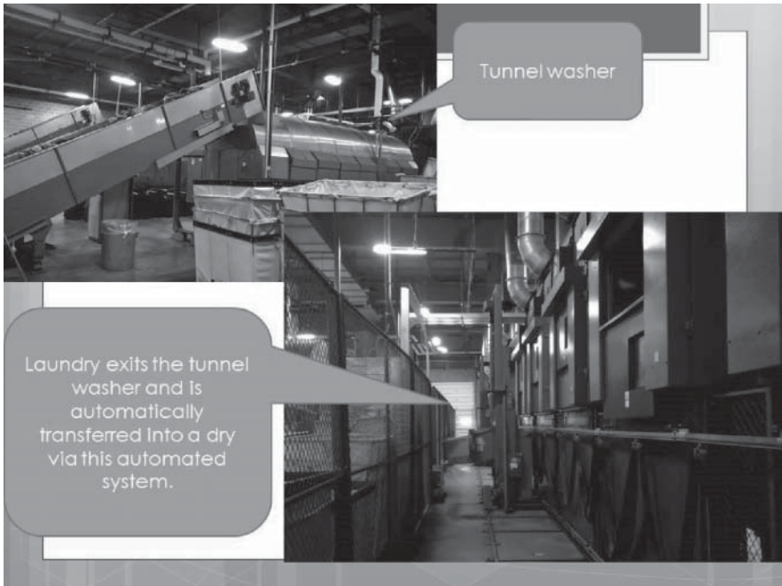
Figure A.18 Laundry is automatically transferred from the washer into dries
