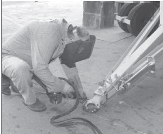
Figure B.9 Before: Welder’s neck and back are in an awkward posture while he kneels on a hard surface
