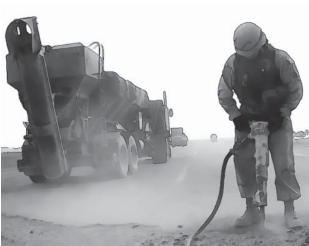
Figure 16.24 Builder from Naval Mobile Construction Battalion Four Zero breaks apart the asphalt with a jackhammer on a road repair project
