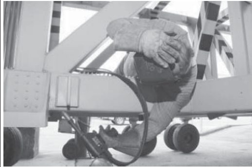
Figure B.11 Before: Welder is in awkward posture to reach beneath work piece
