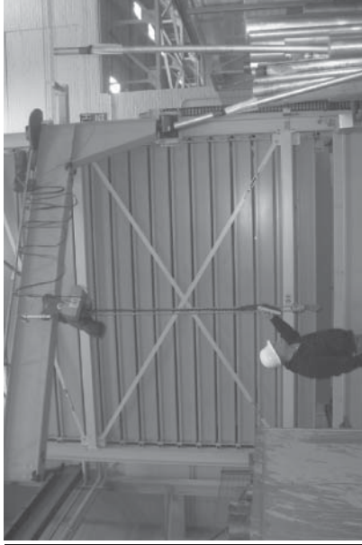
Figure B.5 Vertical index unit for round stock has security access codes for level one stock and incorporates a jib crane at New London, CT
