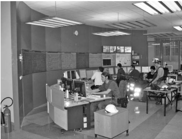
FIGURE 8.8 After the rebuild in 2005, the new control room has a combination of large displays on the wall and a number of small screens for the operators.
