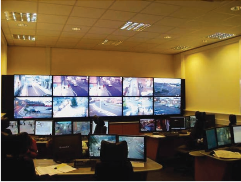
FIGURE 4.33 CCTV surveillance control room for a city centre.
