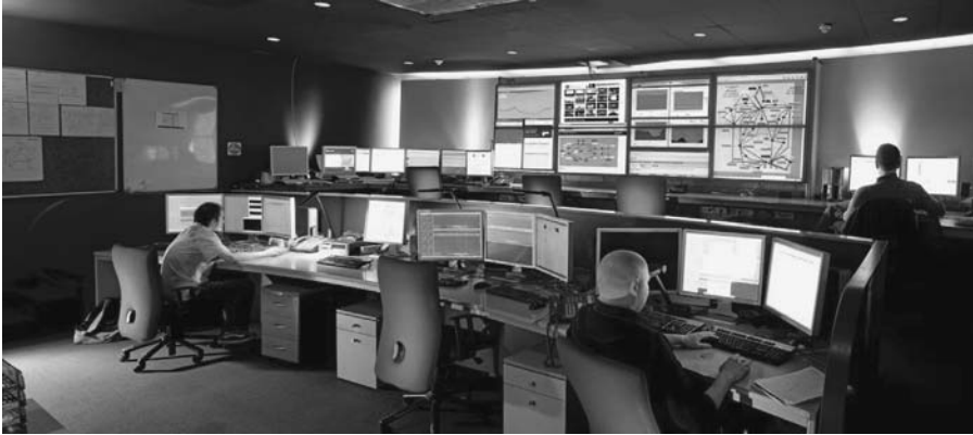
FIGURE 4.33 CCTV surveillance control room for a city centre. (© eyevis-guillaume czerw. With permission.) (See colour insert.)
