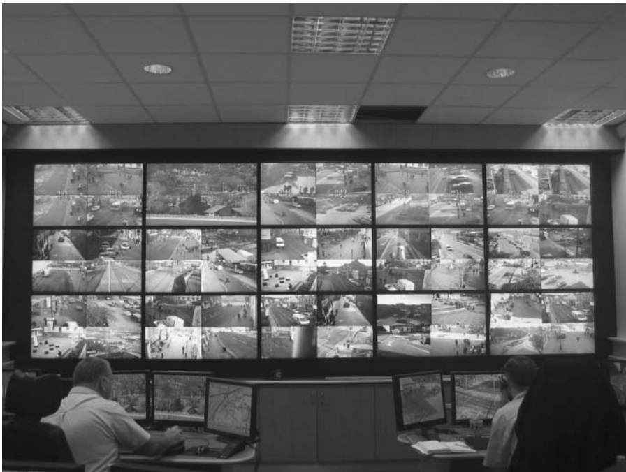
FIGURE 4.32 Control room with an LCD wall, graphics controller, and wall management software. (© eyevis-guillaume czerw. With permission.) (See colour insert.)
